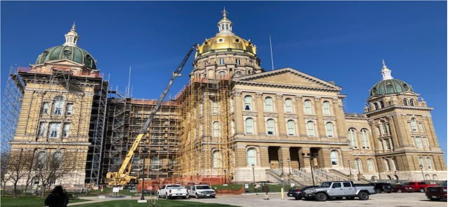
Renovations continue this week on the four smaller Capitol domes. (Photo by The Capitol Group)
