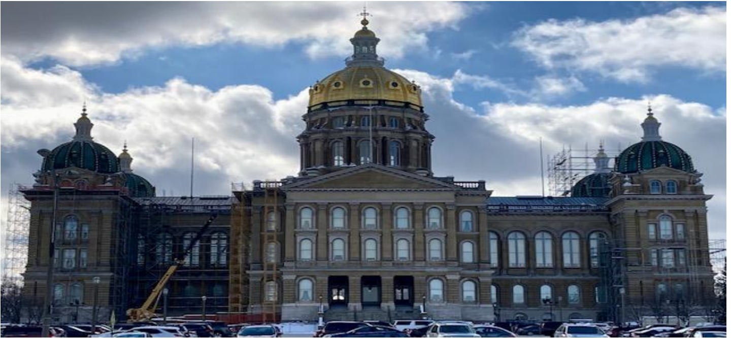
Construction continues on the corner domes of the Iowa Statehouse. (Photo by The Capitol Group)
